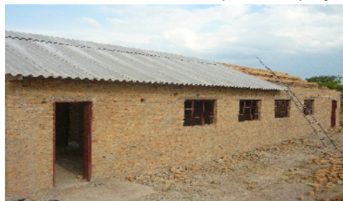
Construction nears completion on the fourth home of the holistic village of Operation Orphan Rescue Zimbabwe.
